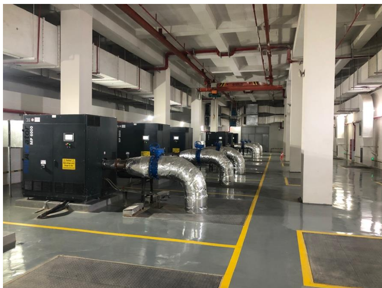
Figure 3: Six Pillaerator Magnetic Bearing Turbo Compressors, Installed in the First Wastewater Treatment Plant of Chengdu Tianfu New Area
